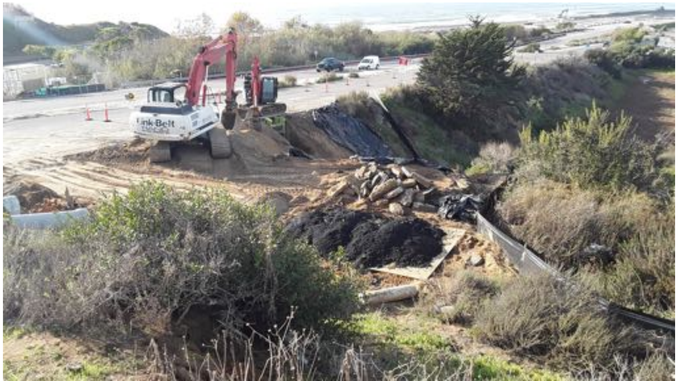
Figure 10: New construction east of HWY101 into Batiquitos Lagoon. This work was interrupted by the Regional Water Quality Control Board.
