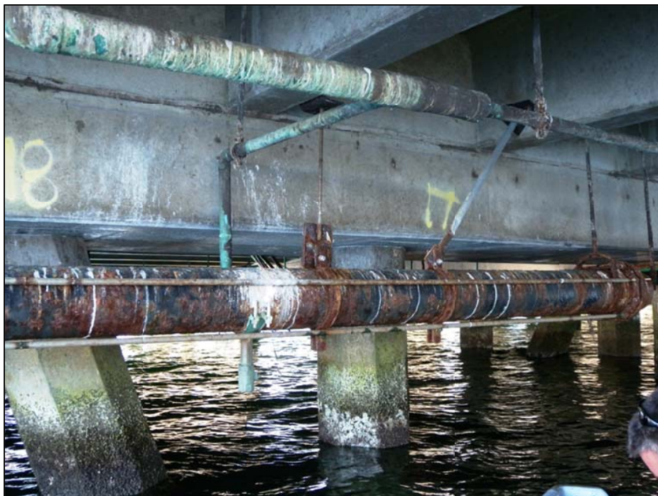
Figure 4-110. Pier with water pipe located below deck. The pipe and hangers may not be designed for wave and current loading.
