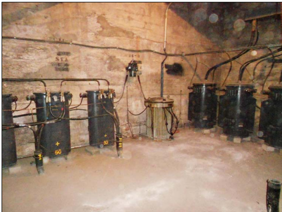
Figure 4-121. The photo shows an electrical vault with older equipment that has exposed connections and is susceptible to flood damage.
