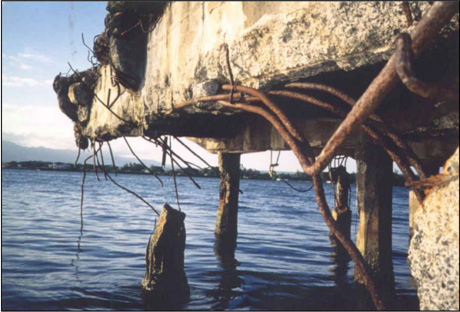
Figure 4-113. Waterfront structure that has excessive deterioration from chloride contamination and corrosion of the reinforcing steel (Courtesy Blaylock Willis and Associates).
