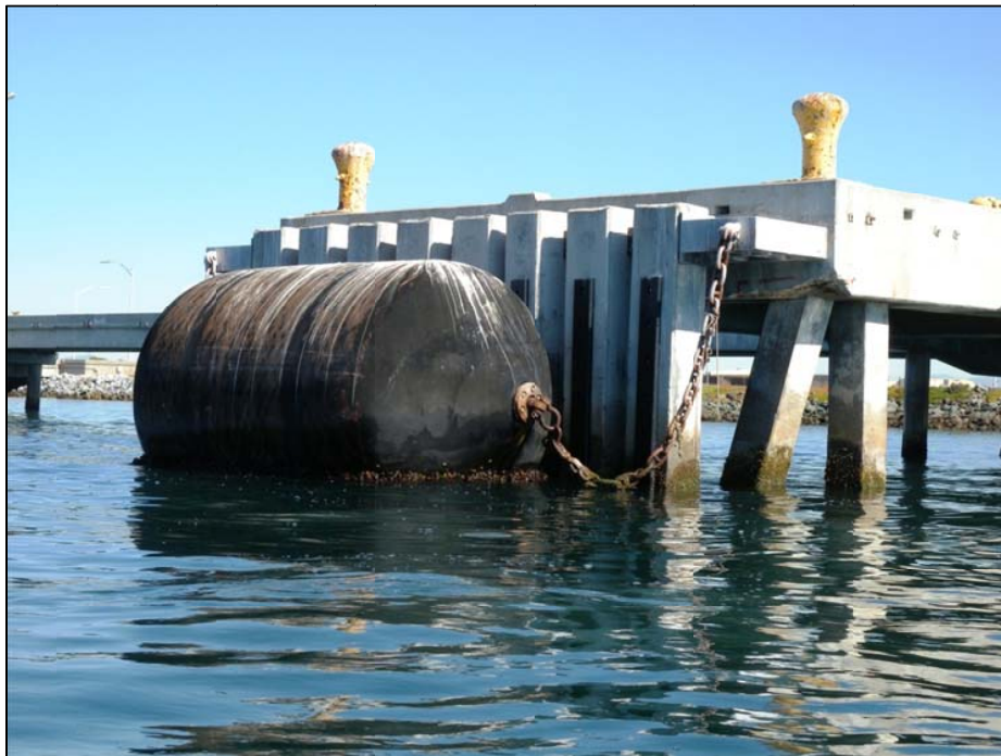
Figure 4-104. Typical pier fender system with floating fenders and concrete reaction piles at a close spacing for bearing.
