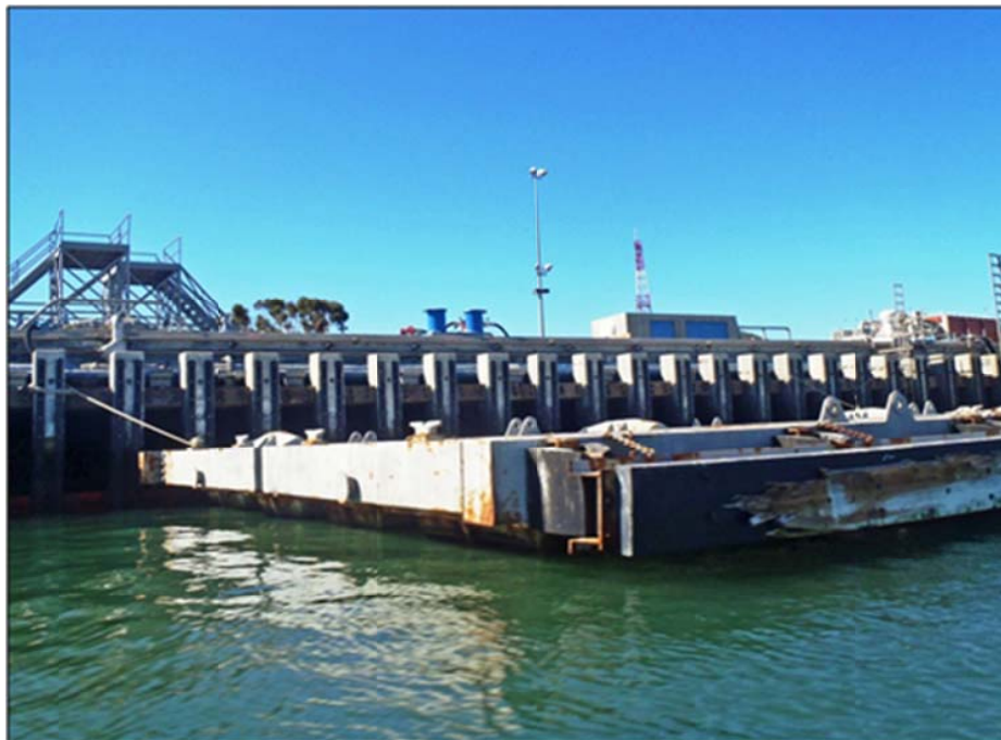
Figure 5-254. An aircraft carrier separator is a floating platform that provides clearance between the aircraft carrier and the wharf fender system, shown moored at Carrier Wharf Berth Kilo, NBC.
