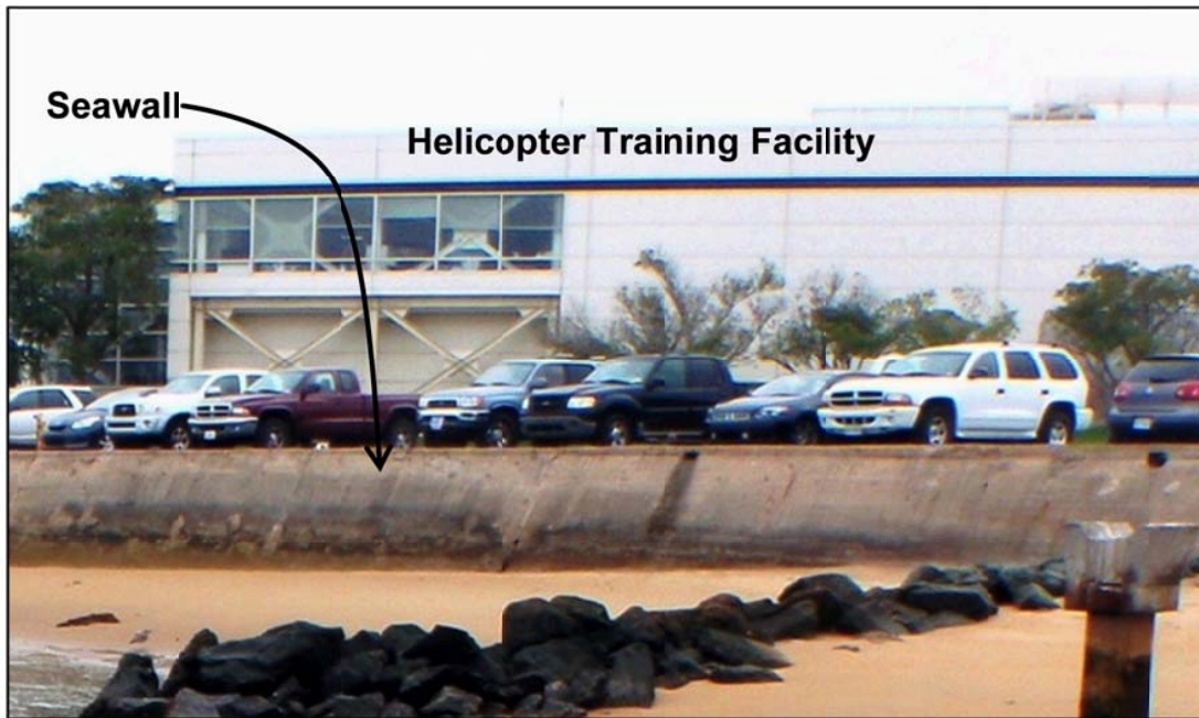
Figure 5-238. View from San Diego Bay looking southeast at the seawall that protects Moffett Road and the Helicopter Training Facility.
