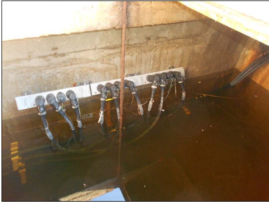
Figure 4-120. The photo shows a below-grade electrical vault partly full of water. A connection panel is visible above the water. The vault remains operational.
