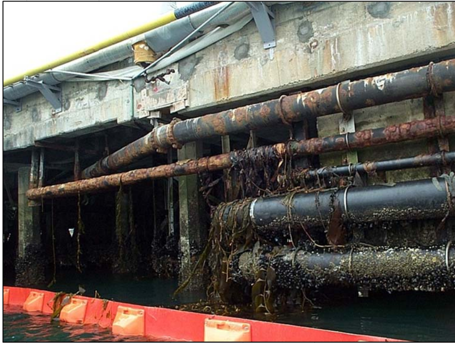
Figure 4-109. Pier with utility pipes located below deck in the tidal zone. The pipes are submerged during high tides and collect kelp and other debris.
