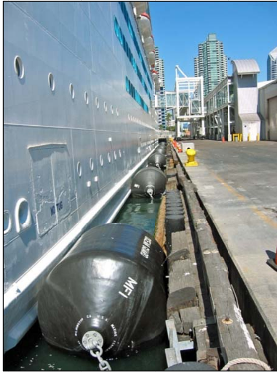
Figure 4-105. Foam filled fenders shown at high tide. With less than 1.0-m of SLR, "roll-over" could occur.
