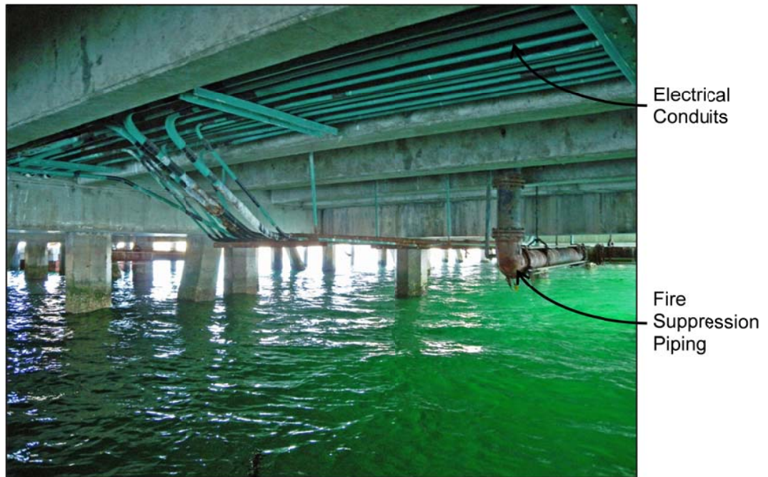
Figure 5-246. The fire suppression piping and electrical conduits at Ammunition Pier Bravo are located below the pier deck.
