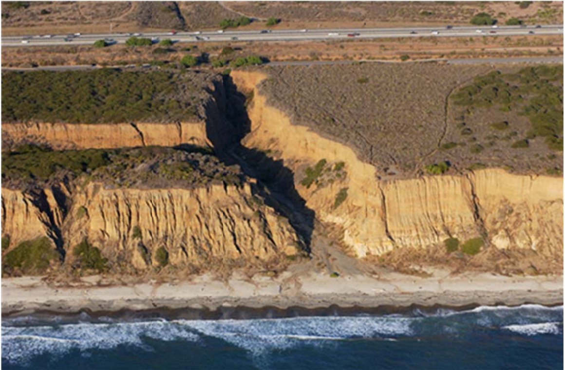
Figure 3-98. Photo of large, deep gully at San Onofre State Beach area of MCBCP (See Figure 3-97 for location; California Coastal Records Project Image 200407227, October 2004; Copyright (C) 2002-2014 Kenneth & Gabrielle Adelman, California Coastal Records Project, www.Californiacoastline.org ).
