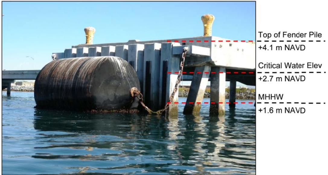
Figure 5-245. View of floating fender and concrete piles at Ammunition Pier Bravo, NBC. This system is vulnerable to “roll-over” with 0.5 m of SLR.
